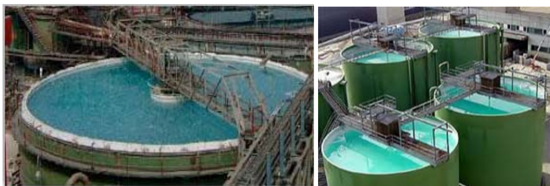
Fig. 1. Brines Purification tanks- Vacuum Salt
